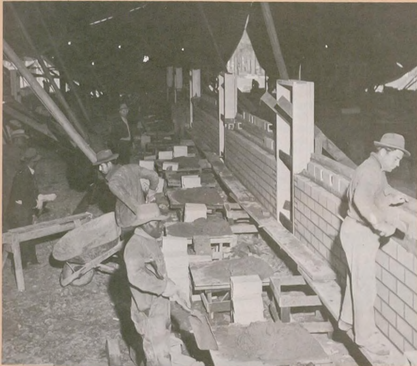
When it became apparent that the rains would continue, Dr. Kemmerer secured a huge tarpaulin, stretched it over the entire construction project, and 160 men worked right on through the rain to complete the building on time.
