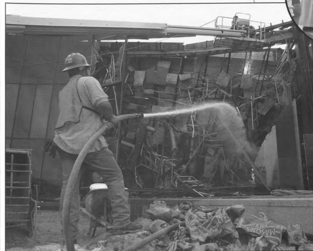
Working together, the welders and fire monitors brought the old library down without incident and started the new home of the M.D. Anderson Library and Honors College immediately after the debris was cleared. Nathan Landsbaum
