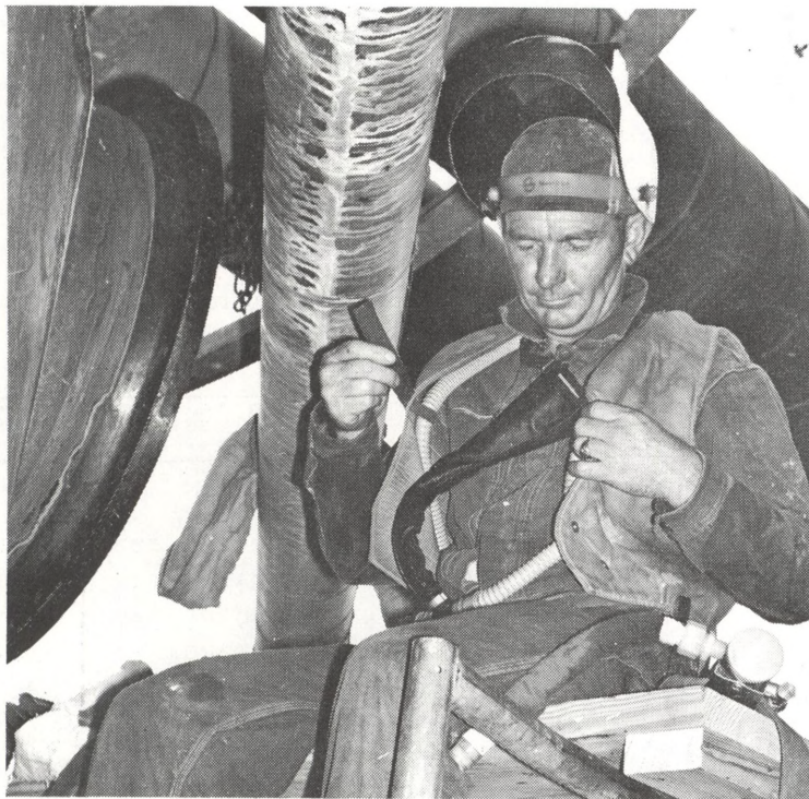
120 DEGREES IN THE SHADE AND COOL, MAN! THAT'S F. L. Shoemake, Welder No. 1 suited-out in his air conditioned vest preparing to weld a 30-inch stub on the vacuum flash chamber at Flasher No. 1 while the unit is running.
