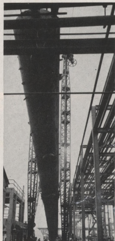
Chemical's tallest column begins its difficult climb toward the skies. It will produce propylene.
