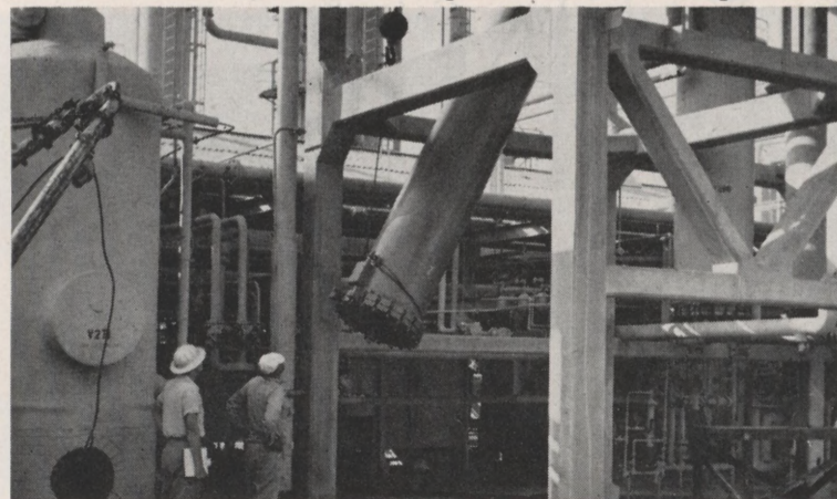
Left, F. M. Stribling, Project Engineer in charge of converter installation in M Plant watches as one of the converters is hoisted into place. When completed the unit will house four converters which will aid in the production of DAA, HG, MIBK, and MIBC.
