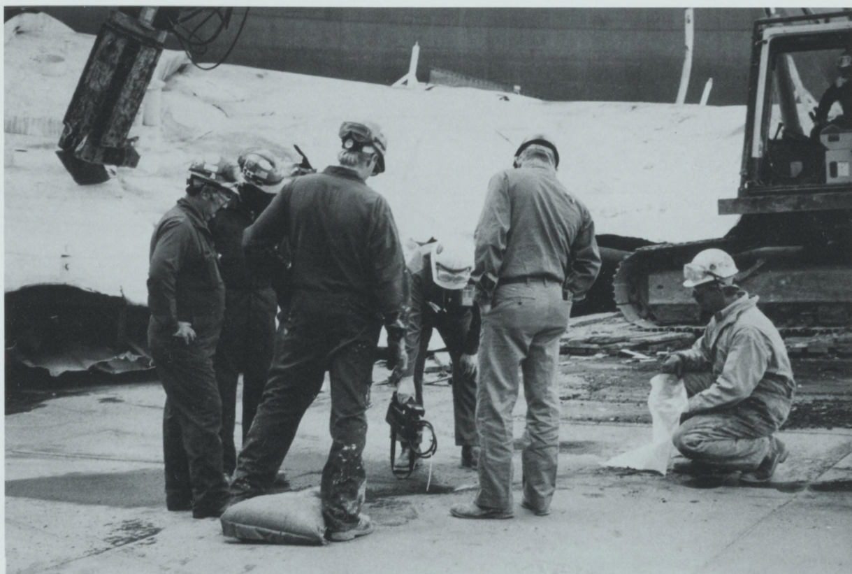
John Flint, Health & Safety; Robert Poye, Tank Maintenance; and CB&I contractors scan the floor of tank A-327 for possible hydrocarbons as a set of dinosaur-like hydraulic shears behind them pauses from cutting up the tank's flood-damaged floating roof. A-327 is 196 feet in diameter, 56 feet high and has a capacity of 300,914 barrels or 12,638,388 gallons.
