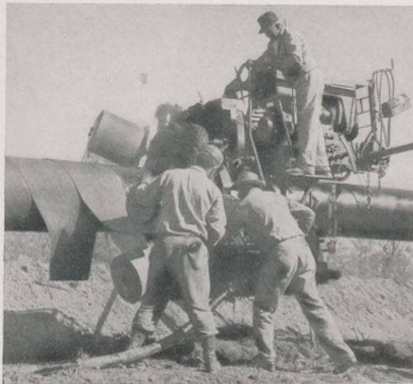
The line is then wrapped with fiber glass to reinforce the coating and an outer wrapper of asbestos-felt provides added mechanical protection. Every inch of the line is then examined for defects.
