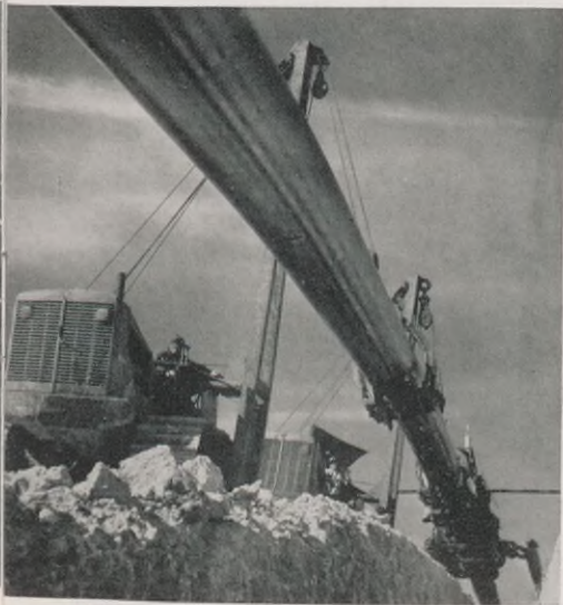
Caterpillar tractors hold aloft a section of the huge pipe line so that it can be cleaned and primed with a protective coating of coal tar.
