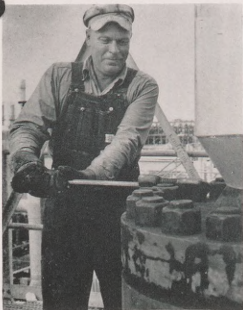
BUTTONING UP —With reactors filled with catalyst the tops and bottoms were bolted shut, above. At this point, months of preparation were nearing an end.
