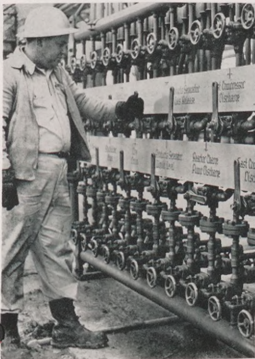
SAFETY FIRST —The panel, shown below, is for remote control of the emergency drop out system. It can open and close valves throughout the plant.
