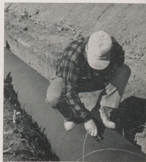
Examiners enlarge each defect with a knife so that it can be detected easily by the repair crew.
