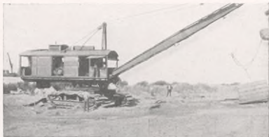
Dredge laying its own road—Agent J. W. Mitchell of El Paso Station and son in the distance
