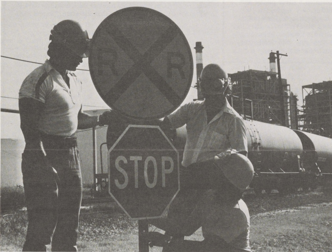
GETTING IT STRAIGHT - Several members of the DPMC railroad crew recently installed one of the new warning signs at this spot near the Tank Farm Control House. From left to right are, Mike Burgess, Paul Saunders and Joe Ramos. The new warning signs, specially designed for industrial use at DPMC, will be installed at each railroad crossing in the Complex.
