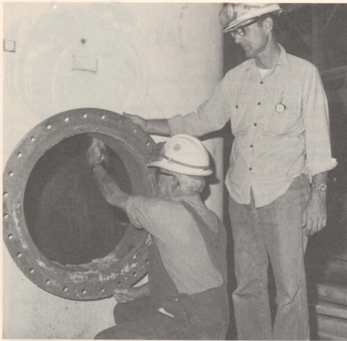
W.E. (Grumpy) Lain, left, and H.L. Siemsen, both Maintenance South boilermakers, install a temporary caustic tank at CA.
