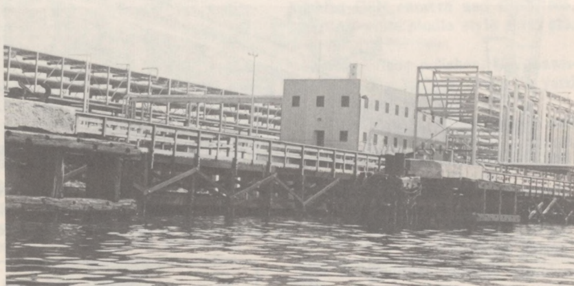
Shown here is the Dock Operations Building, which was occupied for the first time earlier this summer after being under construction since 1978.
