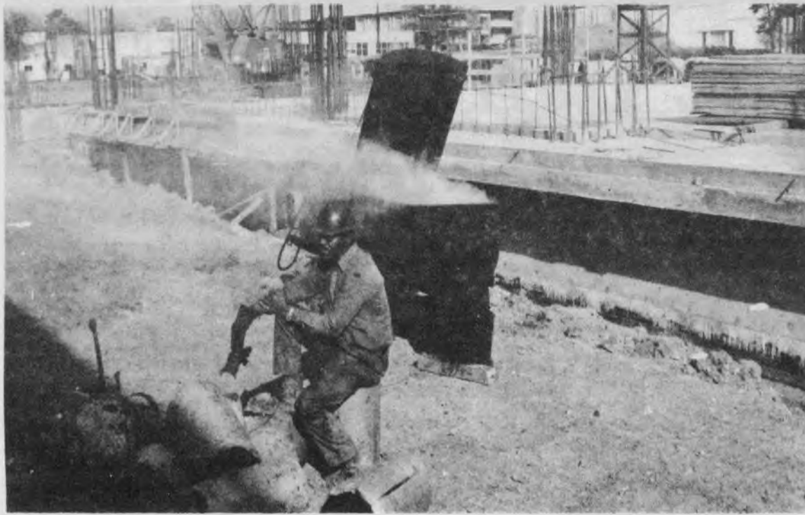
WHILE TAR MELTS and pollutes the construction site of the Classroom and Office annex, this workman placidly awaits the order to throw in another round of the goopy stuff.
