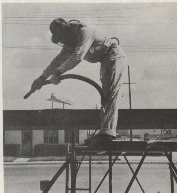
AN INVADER? No! It's Painter No. 1, A. J. Marches, in a protective suit when he was sandblasting behind the Administration Building. Protective suits and head gear are but two of the safety devices used at the Refinery to protect employees from injury.
