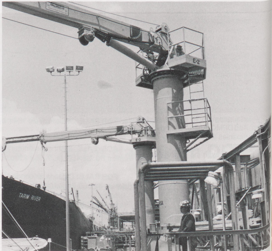
Dockman BUZ MARTINEZ operates one of the 19 heavy-lift cranes used at the Docks to support hoses during liquids transfer between DPMC and vessels in the Houston Ship Channel. As part of the Quality Process, 13 of the cranes are being slowly retrofitted with new components, making the older ones 'good as new'.
