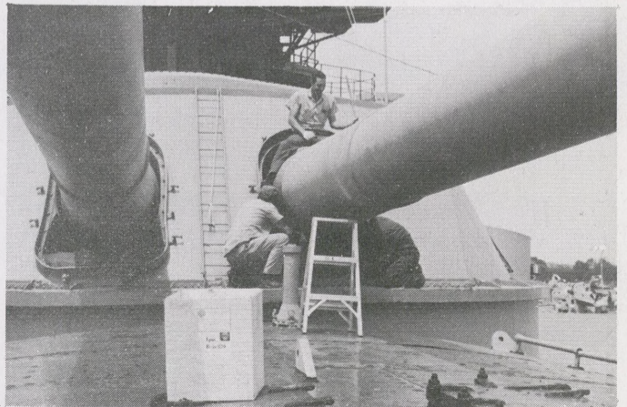
Three crewmen use epoxy resin to seal leaks in the ship's deck and strengthen rust-weakened areas. The resin was manufactured at Shell Chemical Company's plant at Deer Park.
