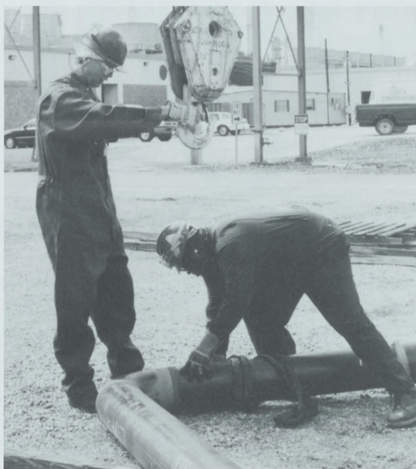
STP—STP crafts persons Jerry Wortham (l) and Don McQueen, working the Lubes' turnaround, prepare to slip a sling over a section of pipe so that a crane can lift it into place.
