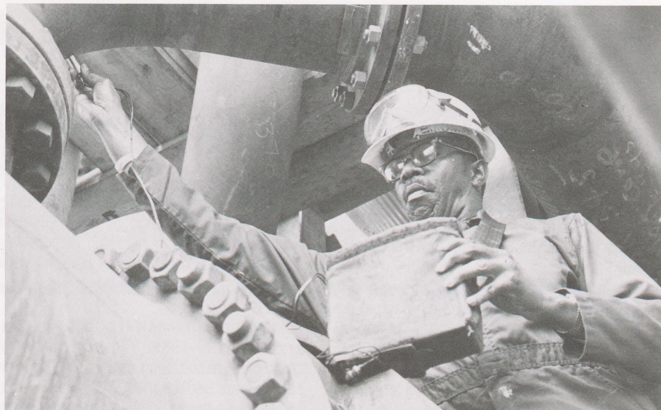
PIPE CHECK...L. O. Jackson, a DU-2 operator, worked as an inspector during the recent turnaround. Jackson inspected newly installed pipe for proper thickness.
