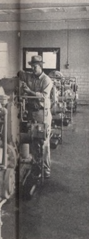
PUMP ROOM at East Houston. These electric pumps can handle 160,000 barrels of crude a day
