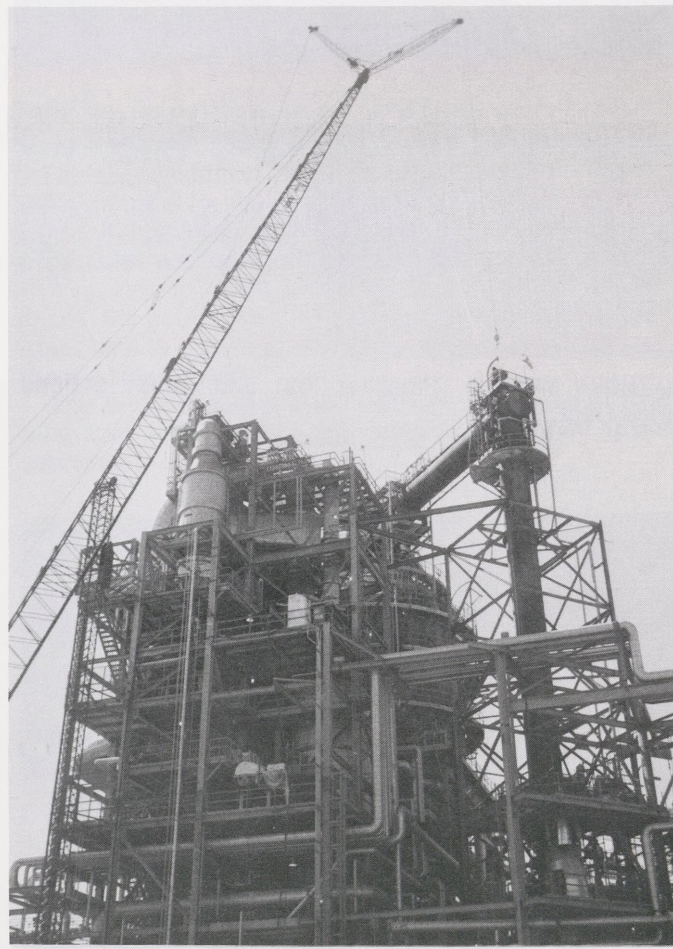
...to the bottom. Quality efforts involved in the planning helped the maintenance work progress safely and efficiently.
