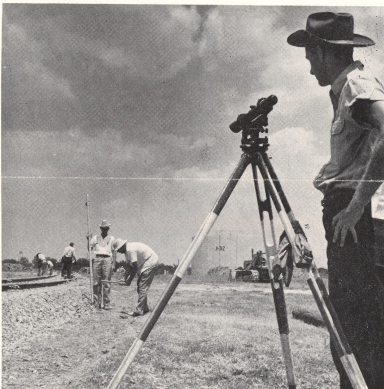
Transitman J. E. Mulare, having completed his reading, watches P. B. Miller drive the stake, which is a step in setting the finished grades for the new Platformer's temporary railroad spur. F. C. Hager is holding the rod.
