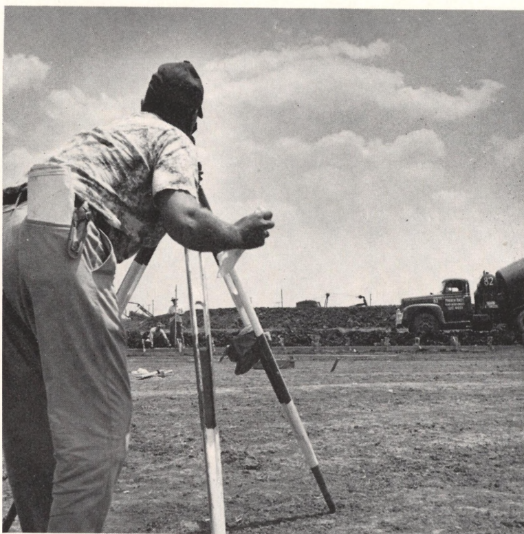
Checking the grade for the concrete ring that is being poured for the new 250,000 barrel AP tank. J. J. Morris takes a reading, G. Kuntz sets the stake and P. B. Miller holds the rod.
