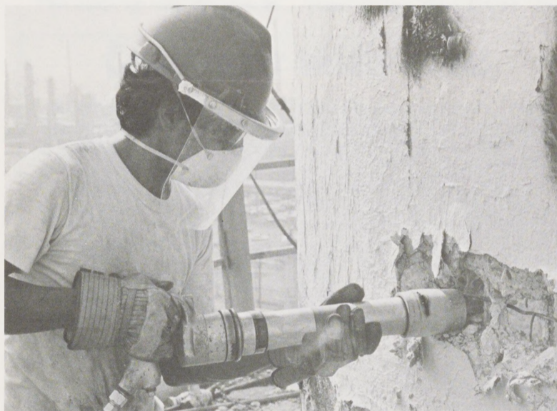
VIEW FROM THE TOP —Crews work from the "doughnut" atop the towering Power Plant 1 stacks, using air hammers to chip away the concrete which falls into the stack and is collected at its base. Despite the grueling labor, the stacks are dropping an average of 16 feet every day.
