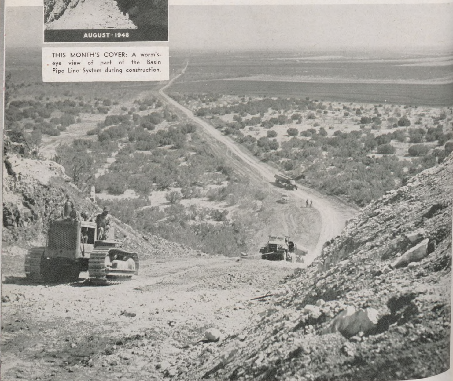
The truck trailer must negotiate the back roads of the West Texas plains. When hilly country is encountered, the weight of the pipe makes it impossible for the truck unit to make the grade under its own power. Then, caterpillar tractors must lend a hand.
