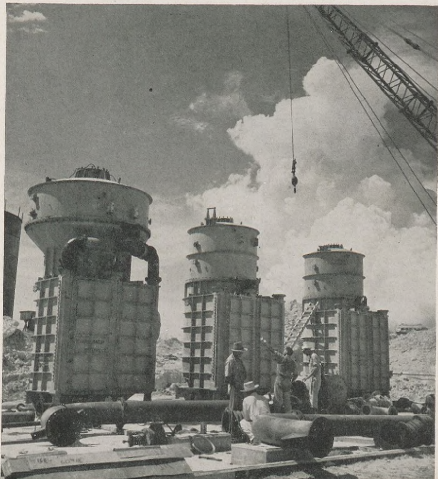
Below. The salt water evaporating plant which is used to convert sea water for domestic and industrial use.
