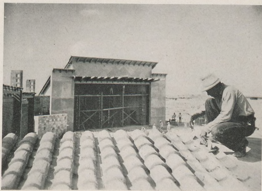
The open-air theater is made of locally produced hollow concrete blocks and has a seating capacity of 1,200.
