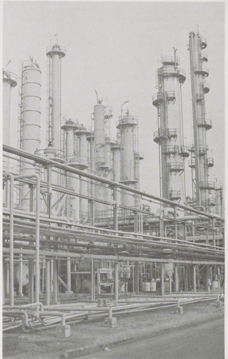
These lofty IPA columns are a familiar landmark in the DPMC skyline. Three sets of columns work together to produce acetone feed stock and "prime" IPA that later becomes finished IPA.
