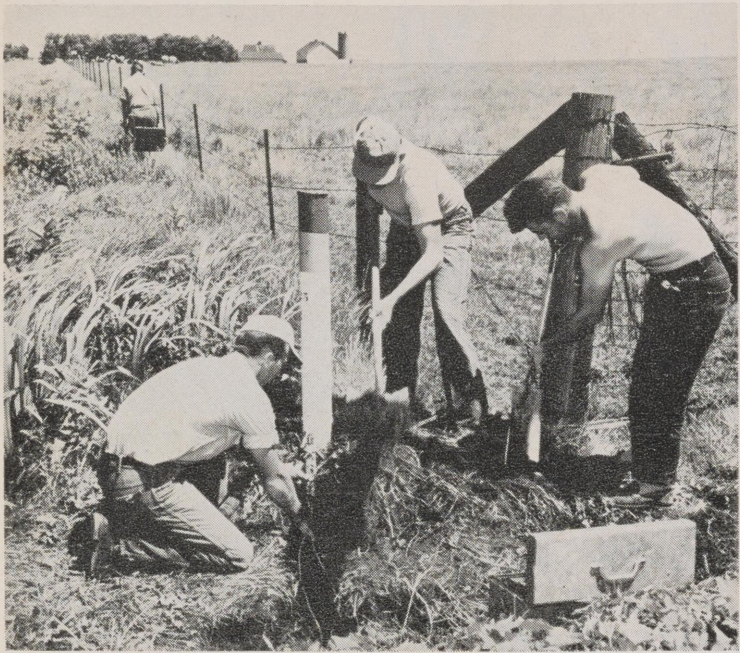
GOODBYE CORROSION —A corrosion Prevention and Mitigation crew plants magnesium bars along the Products Pipe Line's North Line out of Wood River, Illinois. These Magnesium bars, buried in the earth and connected by means of copper wire to the pipe line which is located underground about five feet from the marker post, help prevent or arrest electrolytic corrosion.
