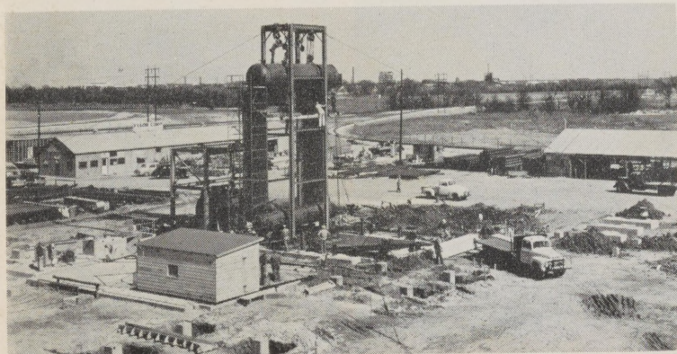
VIEW OF NEW Boiler House area looking North East shows the steam and mud drums in place. This boiler is No. 2-3. The second boiler will be No. 2-1 and will be erected on existing foundations where the boiler makers change house now stands.
