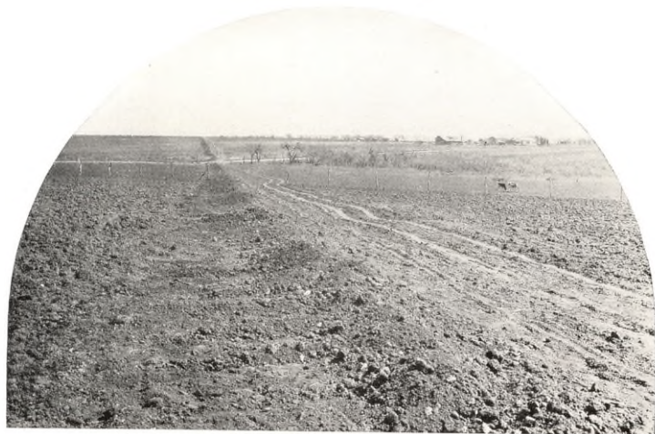
Part of the West Texas Pipe Line After Laying of Pipe and Backfilling
