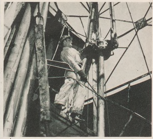
Hazard: Falling. Prevention: A safety belt attaches the derrick man securely to his perch high on the monkey board of a drilling rig.
