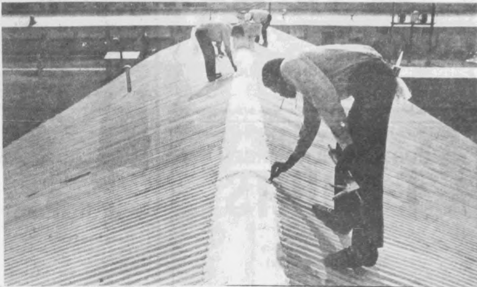
This UH roofing crew resembles a team scaling Mt. Everest. The crew, (bottom to top) Clarence Mosley, Dewayne Bruns, and Irvin Davidson, were sealing recently-driven nails on the North Office Annex roof.
