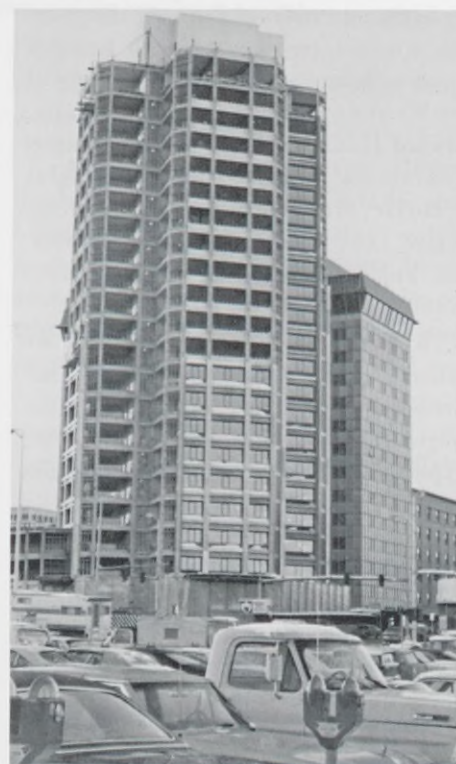
ANCHORAGE-WESTWARD — Towering above the Anchorage skyline the 22-story Anchorage Westward tower addition readies for its early May opening. When completed, the tower structure will be the tallest in all of the State of Alaska.
