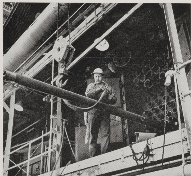
ANOTHER FURNACE TUBE is ready to be pulled into its slot as Boilermaker No. 1 E. G. Suhr removes the strap which was used as a cradle to lift the long tube into position. Removing, replacing and repairing these tubes is just one of the many jobs which must be accomplished before the Cat. Cracker can go back on stream.
