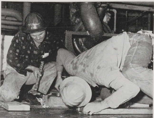
STANDING ON YOUR HEAD is recommended by some yoga experts for relaxation, but it is also sometimes a necessity in order to get a job done during a turnaround. Here T. C. Cardwell, Machinist No. 1, drives a wedge while under the close scrutiny of Machinist Helper No. 1 I. E. R. Crofoot.
