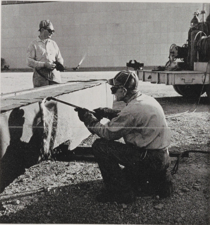
BURNING AWAY DAMAGED portions of grid beams is one of the many jobs the Welding Shop handles during a Cat. Cracker turnaround. Here F. L. Shoemake (left) and J. L. Dykes, both No. 1 Welders, work on one of the mutilated beams, getting it ready for replacement of the damaged portions.
