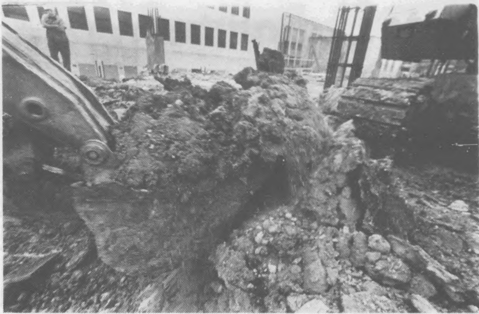
THIS STEEL MOUTH bites the dirt as construction continues for the M.D. Anderson Memorial Library's new wing.
