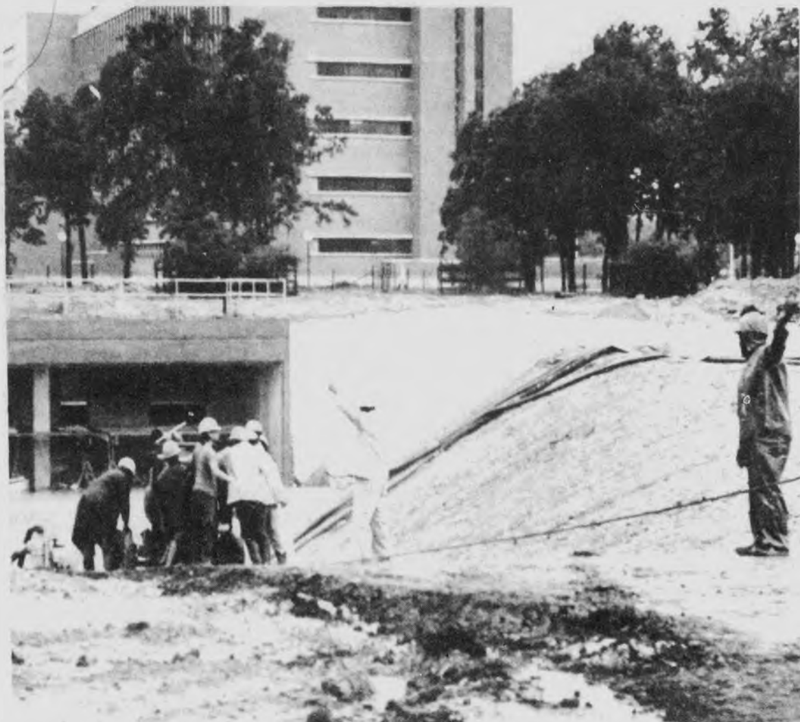
THE TORRENTIAL RAINS collected at the entrance to the UC Satellite site as workmen tried in vain to pump the water out of the underground building. Officials say damage will be estimated after the water runs off. JOAN DUFFY—Cougar Staff
