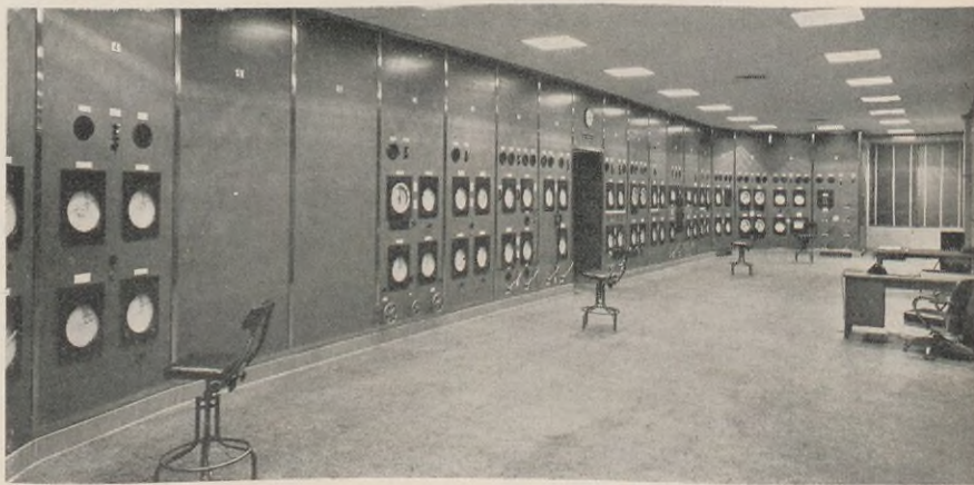
(Above) The modern air-conditioned control room, specially tinted to limit eye strain.
