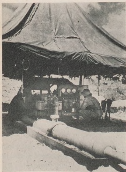
Pumping station of the portable pipe line as actually set up for use in the field. The one here depicted was installed at Camp Claiborne, Louisiana, for the training of soldiers in the Petroleum Supply Section.
