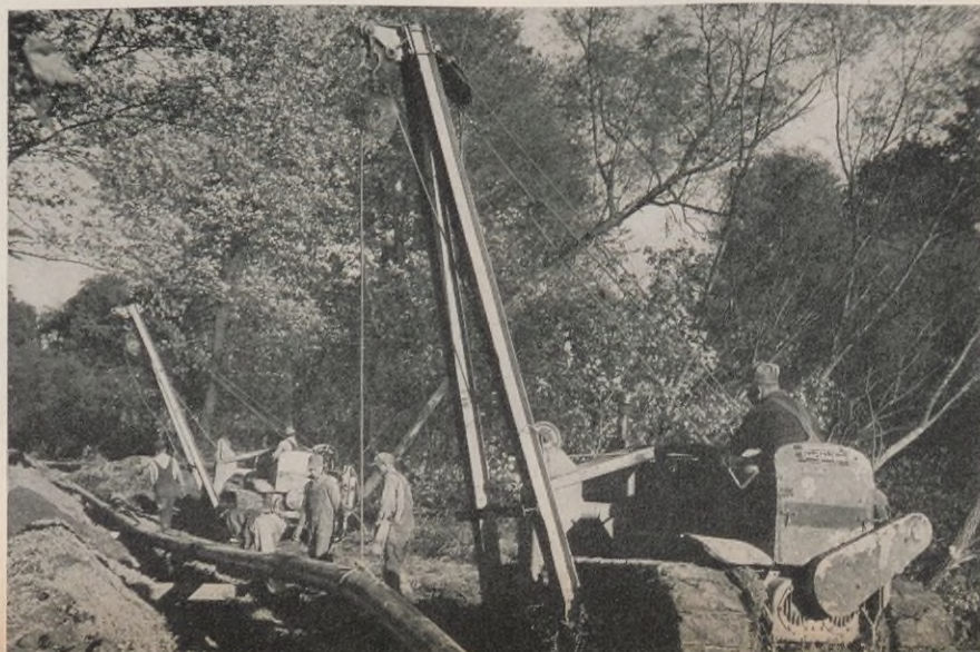
Laying one of the crude lines of the Shell Pipe Line Corporation
