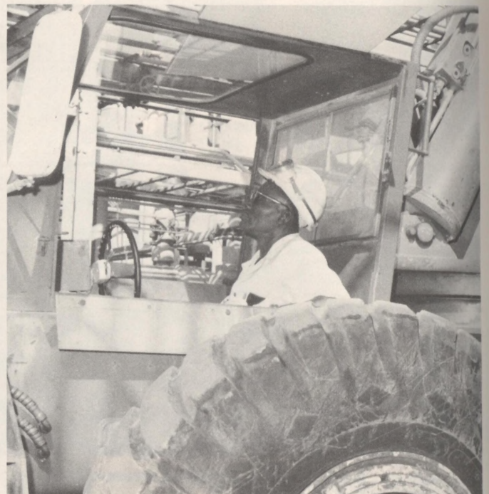
D. Faultry, a South heavy equipment operator, moves his crane closer to a work site at the sniff gas column.
