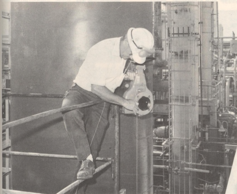
James Hobson, a South pipefitter, checks his measurements before working on piping at the sniff gas column.
