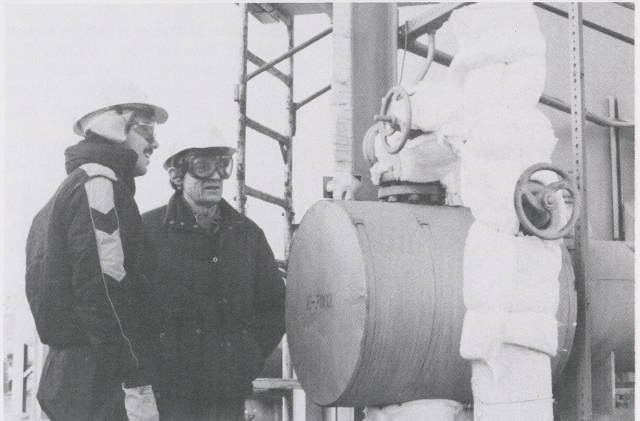
PROTECTING PIPES...Leo Flores, left, Process Engineering, Utilities and Van Huddleson, Utilities, inspect insulation added to pipes at Power Plant-2 as a makeshift measure to combat freezing temperatures.
