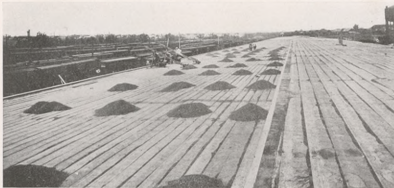
1,200 Squares of Texaco Overlap Roofing 120,000 square feet of Texaco Overlap Roofing applied by Peden Roofing Company to the roof of the new Concrete Cotton Warehouse of the M. K. & T. Railway, Houston, Texas, view showing the roofing applied to the concrete surface, ready for the top coating of asphalt and gravel.
