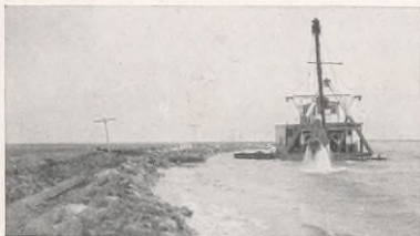
Dredge constructing a section of flood protection levee which also acts as a bank for a fresh water reservoir. The dredge is floating in about 6 feet of water.
