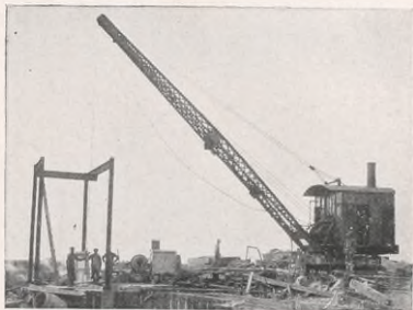
Locomotive Crane lowering pump parts into a pit. The two pumps have a combined capacity of 35,000,000 gallons in a 24-hour day.
