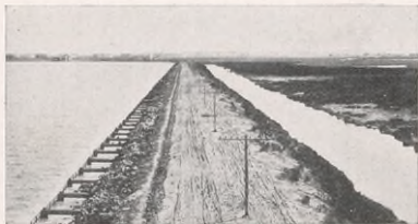
A section of completed flood protection levee. At this point the levee also acts as one of the banks for a fresh water reservoir. The area subject to inundation by flood is shown at the right.
