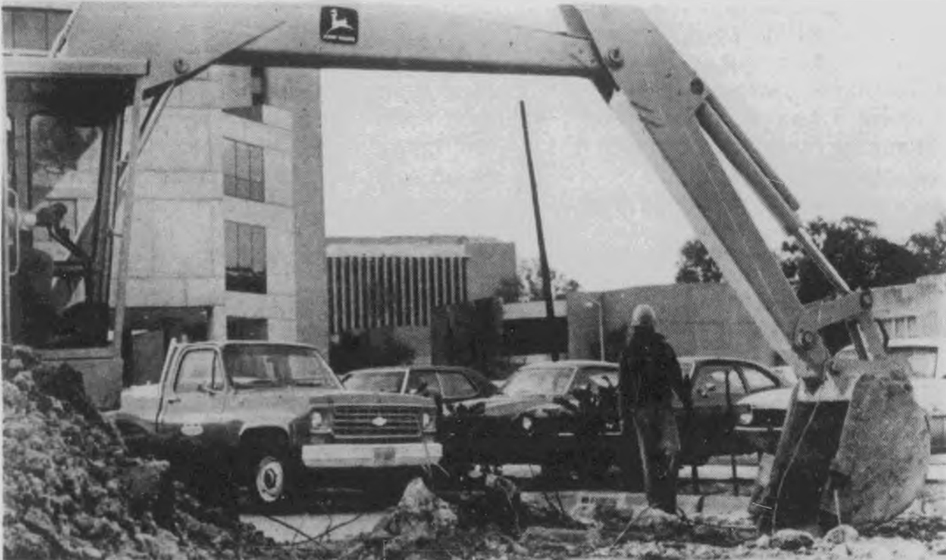
DIGGIN' IT. Mammoth tools aid workmen in the excavation needed to install additional drainage pipes in the area
