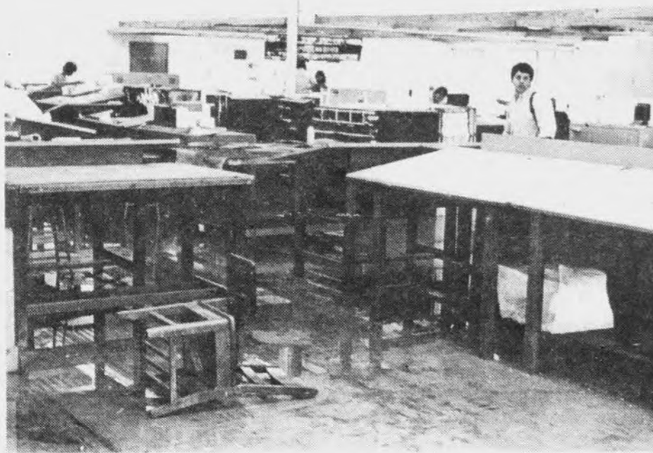
When it rains it pours. And when it pours, it pours in the Architecture building (above). Yesterday, the rains came through the ceilings of the Architecture lab, library and band annex. (Photo by James Leifeste)
