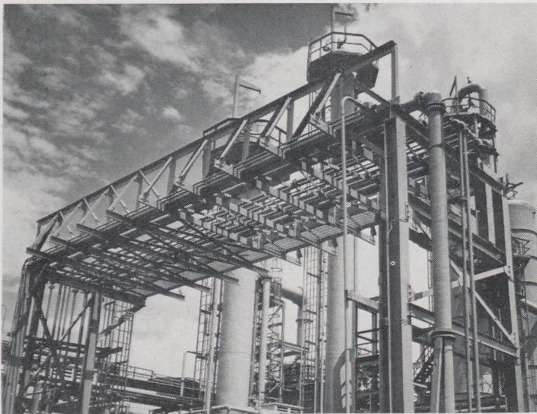
Over head pipeway carries Utility and Process lines to unit.
