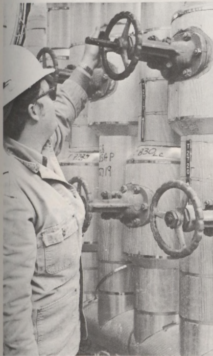
Operator Randy Walker performs routine task of turning a valve in the recently completed ERU-5.
