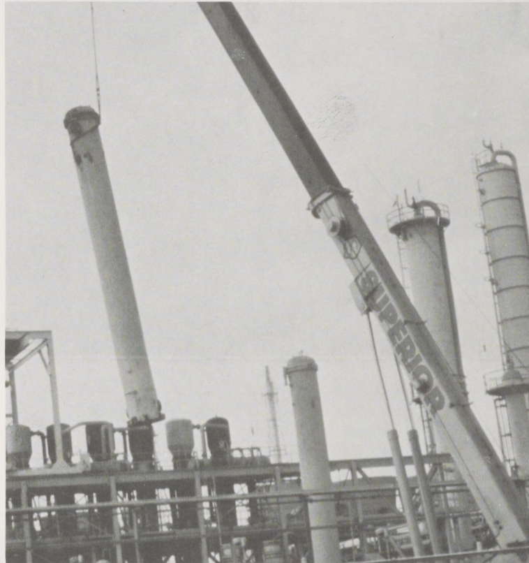
The largest hydraulic crane in the United States lifts an IPA reactor from its base as part of the Complex dismantlement project. The 47,000 pound reactor was one of four removed, each in one piece. The reactor was cut at its base and hauled straight up by the crane, before being loaded on a flatbed truck. This equipment, which was dismantled in late September, was to be sold as used equipment. The dismantlement project, which began in August, is approximately 15 percent completed.
