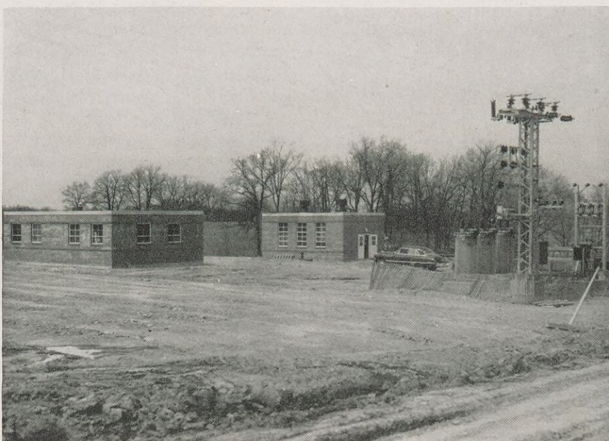
The new booster station at New Douglas, Illinois, (shown at right, during construction) is one of four which can be operated by remote control from the Chief Dispatcher's office in New York City. The control building is at left, the pump house in the center, and the electrical substation at right.
