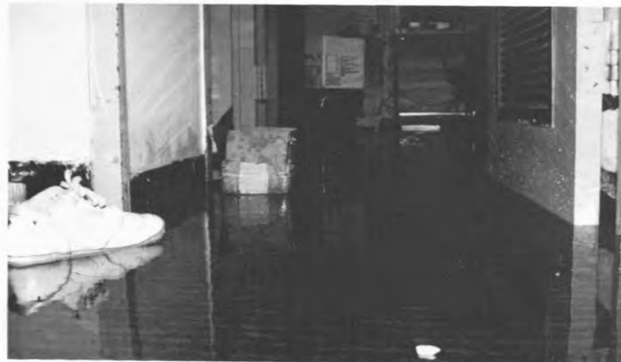
A Soggy Situation. The after effects of the explosion that got third floor Settegast residents all wet! Photo by Danny Rodosovich.
