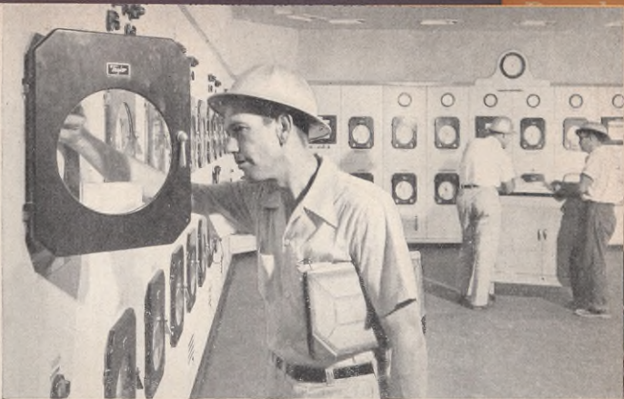
IN THIS CONTROL ROOM for the ethylene oxide unit at the Port Neches plant, one of Jefferson Chemical Company's highly trained operators sets a gauge. Pilot plant for this unit was originally set up in The Texas Company's laboratories at Port Arthur Works, was later moved—as it appears in the photo left—to Jefferson's Austin Laboratories
