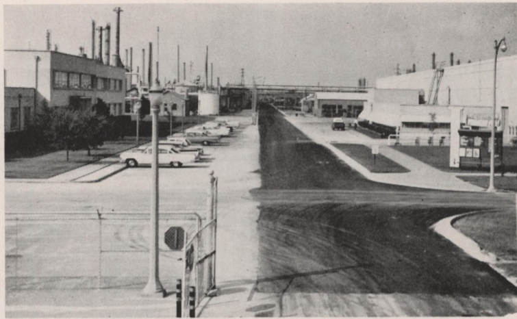
WEST 10th STREET at the Chemical Plant may have looked like an avenue in Venice at the height of the summer rains, but after the rebuilding and resurfacing was completed the road can now accommodate heavy trucks and cranes.
