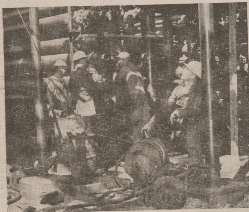
Men in background are Boilermakers installing screwed collars on tube ends of a concentric tube type heat exchanger. Left to right are: unidentified helper, M. L. Neel, boilermaker, 2nd class and M. D. Cothran, boilermaker 1st class. In foreground is J. M. Willard, pipefitter, operating trigger hoist, hoisting pipe to top of fractionating column.
