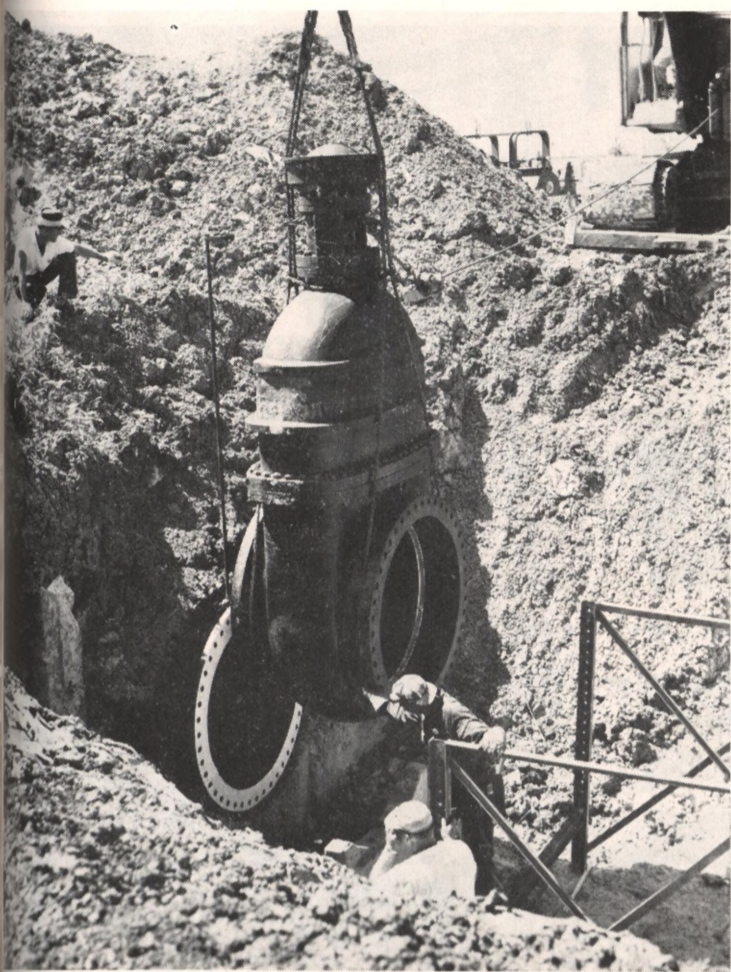
48-inch gate valve is being set on the water system's main head to enable Shell to tie-into the water supply from Lake Houston.
