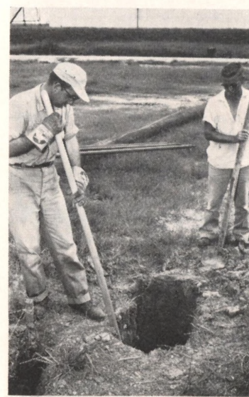
C. L. Easton, left, and B. R. Jackson finish digging a hole in which a power light pole will be installed.
