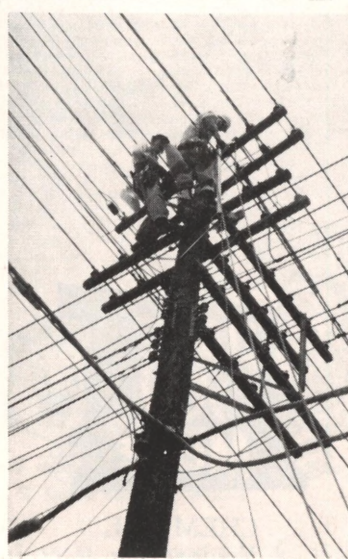
J. C. Johnson, left, M. W. West complete a maintenance job atop one of many power poles in Houston Refinery.
