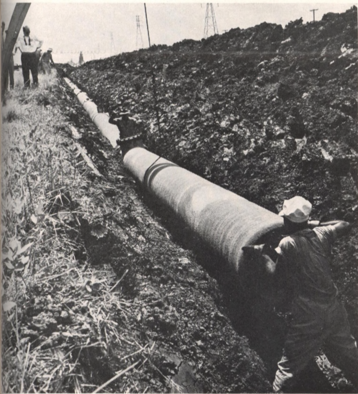
A section of the 24-inch treated water line that will transport the water from the treatment plant to the reservoir is shown above.
