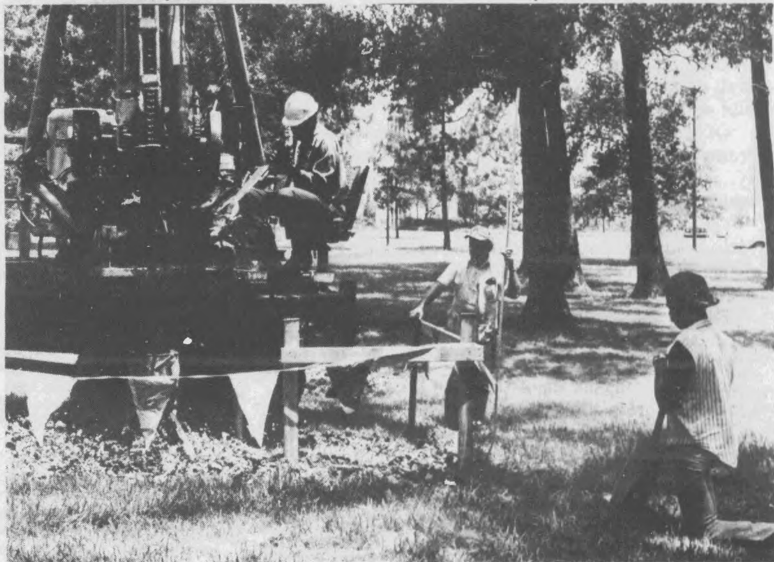
Workers of the Homer Weaver Construction Company dig post holes for the new Eusan activity platform, a 30 x 26 foot stage being built
