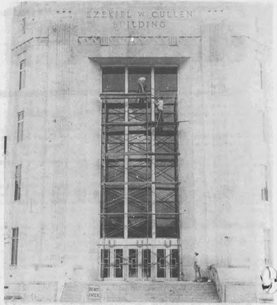
THEY'RE STILL AT IT. Workmen are replacing the window panes that were broken during the first installation with new ones.
