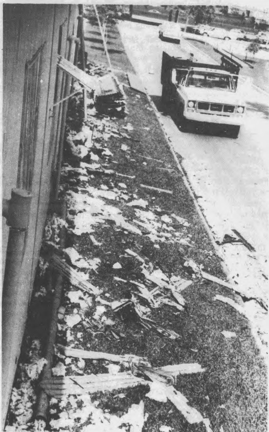
REPAIRS are being made on the Art Annex building, which was damaged by a car wreck. Insulation and pipes were scattered on the ground. TONY BULLARD—Cougar Staff
