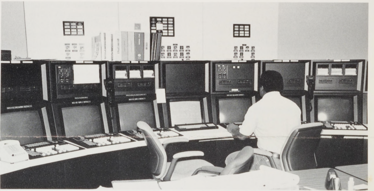
NEW CONTROL ROOM - John Broussard, one of Lube Manufacturing's "crossover" coordinators, (Not pictured is Fil Saenz, Lube's other coordinator) monitors the processes of two units now controlled electronically in the new control room. The screens are replacing the pneumatic controls found in the department's other three control rooms which are also scheduled for crossover.
