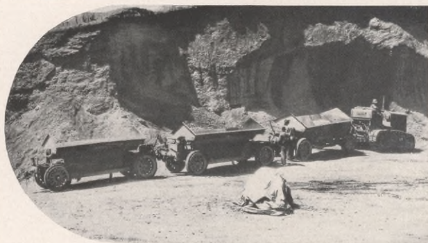
A Volcano Helps Make a Highway: An Old Lava Bed Near Puebla, Mexico, Yields Material for Hard-Surfacing Near by Roads
